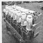
HPU •1-5 subm. pump •3-7 ext. pumps
